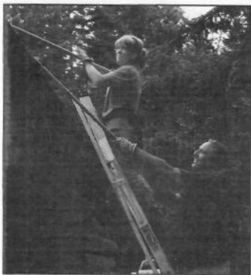
Laurie and Mark Nale remove moss from cabin roof at Kidney Pond during VIP project.
