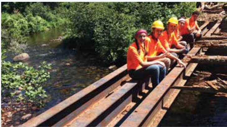
Members of the Patten BYCC crew rest for lunch on the steel structure of the bridge that they demolished and rebuilt over the course of four days.
