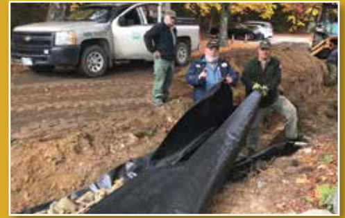
Park staff working together to solve major erosion problems at Katahdin Stream Campground. L to R: Tim Deetz, Gil Moreau, Matt Martin, and Frank George.
