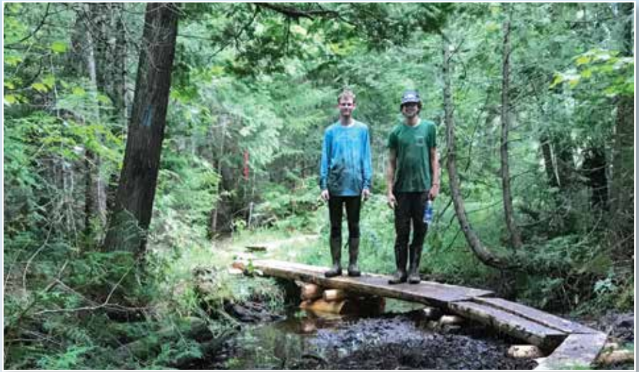
Mike Clark of Millinocket and Kyle McNally of Stacyville with a section of bog bridging they built on the Mount OJI trail during the 2022 Baxter Youth Conservation Corps. – Photo © Greg Friel
