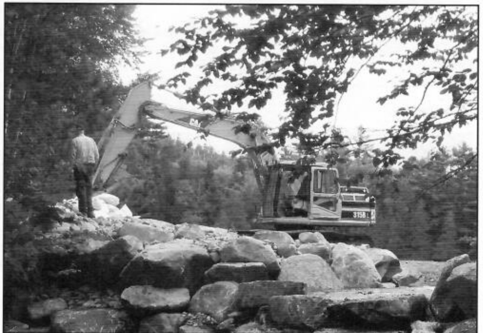
Work shown above in progress on dam removal at the outlet of Abol Pond has been completed.
