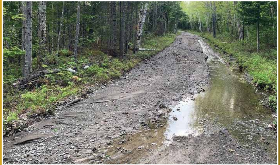
Road damage following an intense 4.5" rainfall event in the north end of Baxter State Park.
