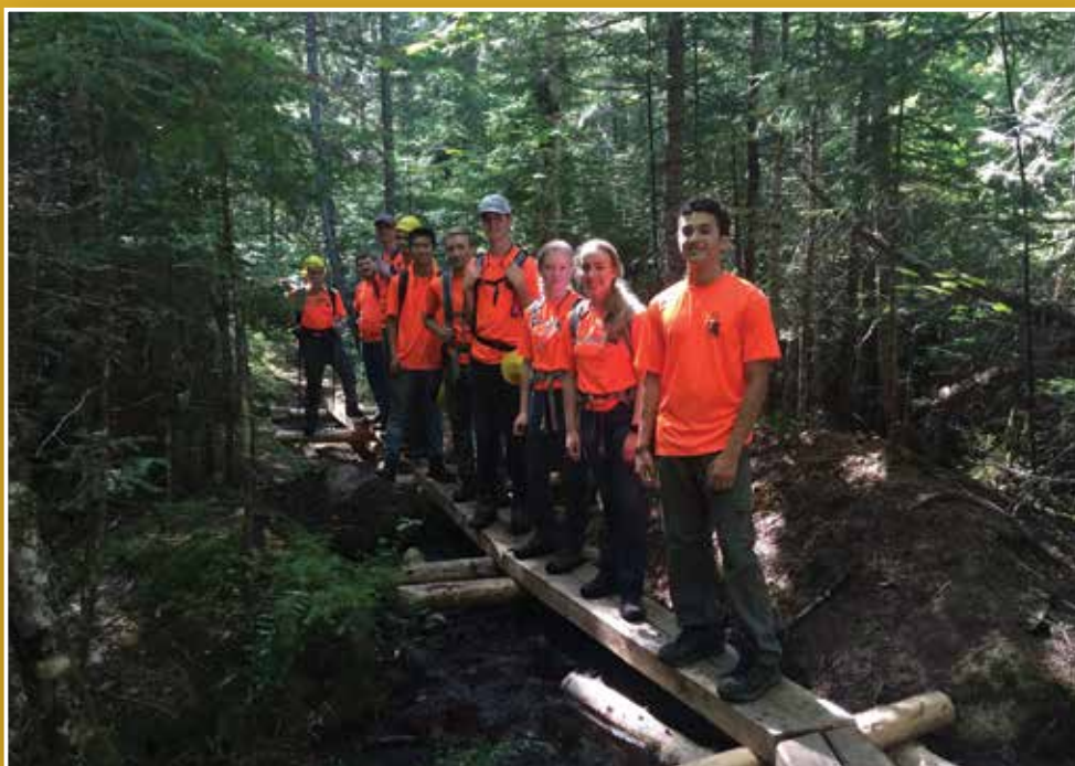
Liz Thibault, BSP Trail Supervisor, planned and oversaw the replacement of this bog bridge carried out by members of the 2019 Baxter Youth Conservation Corps.
