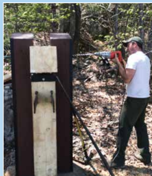
Park infrastructure requires continual maintenance, and sometimes complete replacement. Here, BSP staff are installing a new gate at Matagamon.
