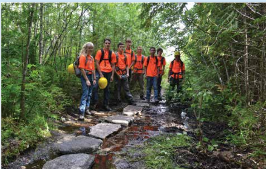
Members of the Millinocket-based crew of the 2018 Baxter Youth Conservation Corps with stepping stones they installed on the Blueberry Ledges Trail. – Photo © Aaron Megquier
