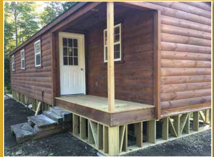
BSP staff are hard at work on building repair and replacement in several areas of the Park. – Photo courtesy of Baxter State Park
