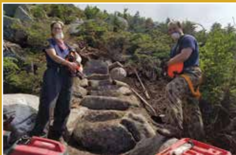
Members of the Maine Conservation Corps building a stone staircase on the new Abol Trail.
