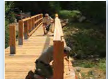
BSP staff installing a new footbridge at Katahdin Stream Campground. – Image courtesy of Baxter State Park
