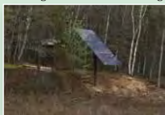
New solar panels provide power to the Togue Pond gatehouse. – Image courtesy of Baxter State Park
