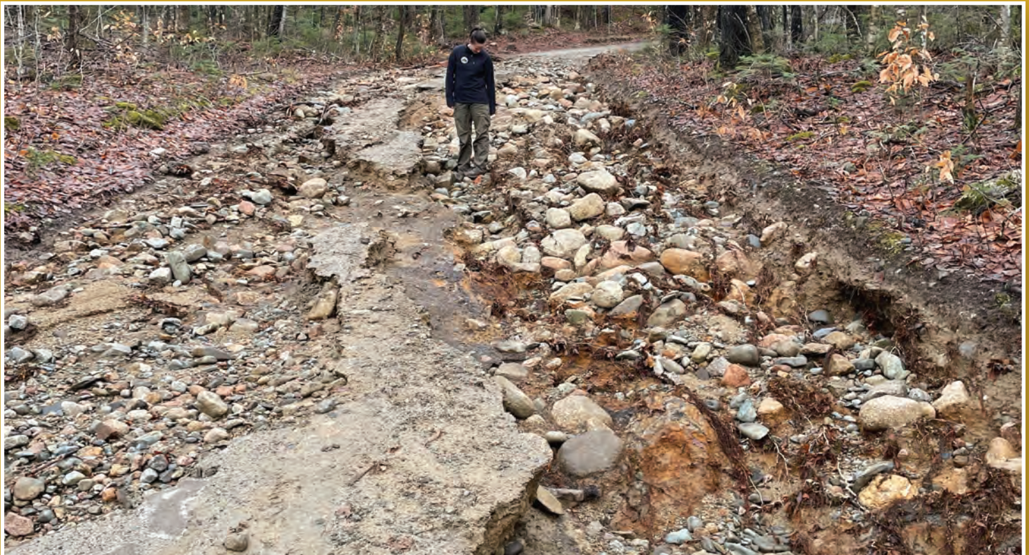
Damage to the Roaring Brook Road following a heavy rainfall event on December 18, 2023.
