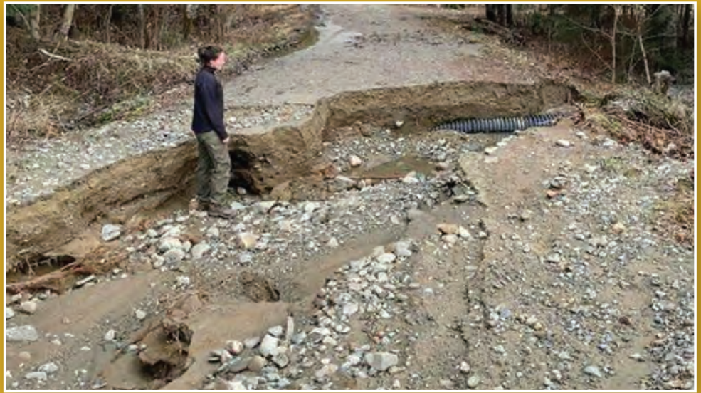
Flooding damage to the Tote Road near Nesowadnehunk Field Campground in December 2023.
