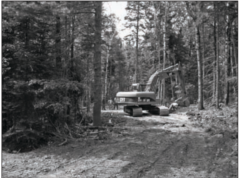
SFMA Park Tote Road connector in the "Forestry Mile" shown under construction here is now complete. — Photo by Park Staff
